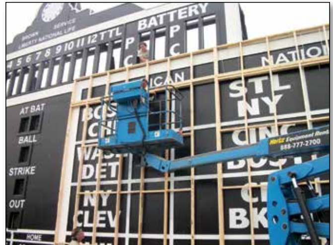
"42" construction department members alter the appearance of Rickwood Field's iconic scoreboard. Courtesy of Friends of Rickwood.
